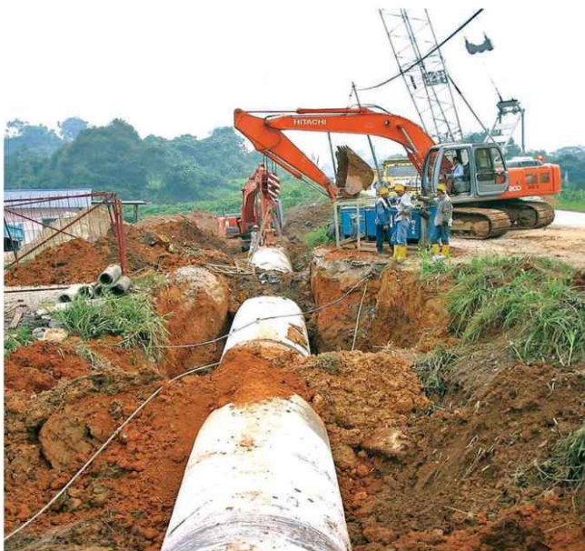
1600mmND Steel Pipeline from Jalan Batu Kitang to Jalan Datuk Stephen Yong / Jalan Batu Kawa Junction, Kuching (2003)
