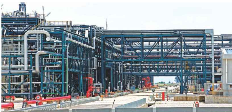
Polycrystalline Silicon Manufacturing Plant for Tokuyama Malaysia at Samalaju Industrial Park, Bintulu (2011)
