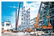
Sejingkat (210 MW) Coal - Fired Power Station, Kuching (1995)
